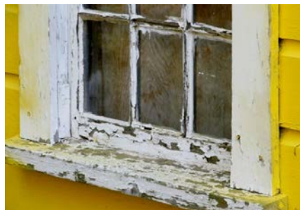
Lead Paint on Old Windowsill
